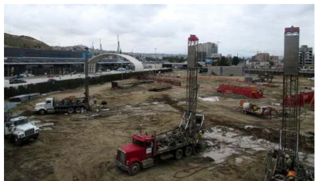
Construction was ongoing at the San Ysidro port of entry in May.
