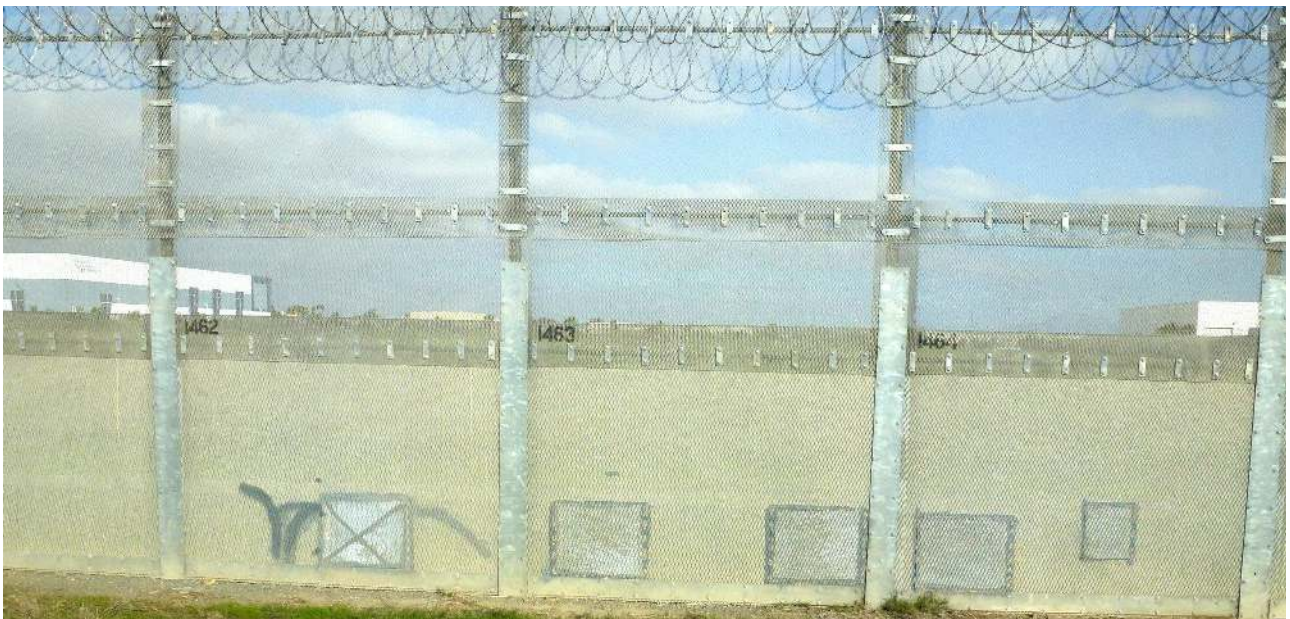
Patches in the San Diego border fence. (Credit: Adam Isacson)
